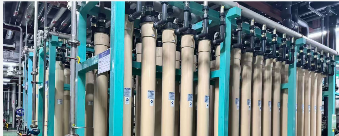
TCL CSOT Reclaimed Water Recycling System
