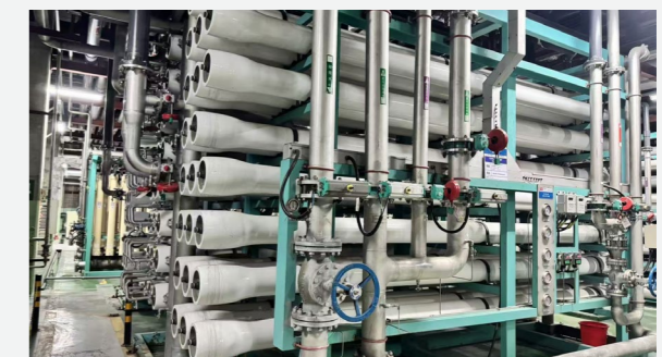
TCL CSOT Water Reuse Equipment
